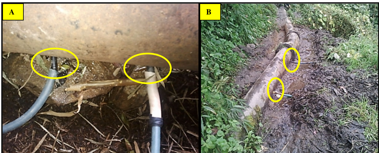
Fig. 7 A andB: Illegal tapping of water in the main transmission line at Alooari and Ganeshgram (Ward no. 1 & 14). Source: DM 2012b
