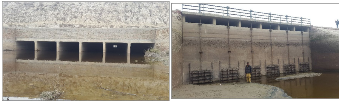
Fig. 10 SB Nullah siphon under SMB Link canal (L); and its escape gates to the siphon
