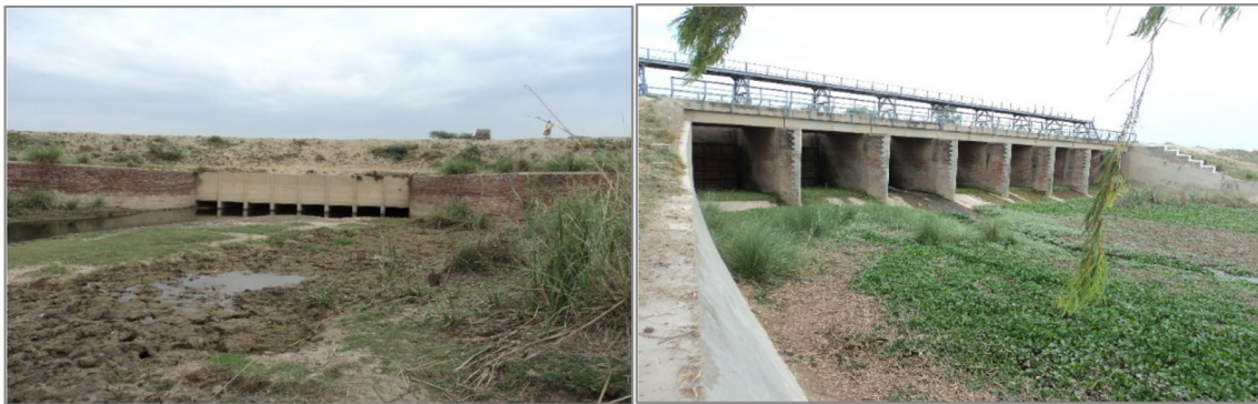
Fig. 8 Sukh-Beas River siphon under BS Link canal (L); and BS Link-I escape to Sukh-Beas (R)
