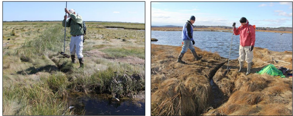
Fig. 2 Left: Creation of runnel by compacting the marsh surface using a handheld tamping tool at the north pool site in 2015. Runnel connected an existing ditch to the expanding pool. Right: Runnel at the south pool site in 2015 after construction. Runnels were created with dimensions of approximately 30 cm width - 15 cm depth and lengths of 60 – 200 cm
