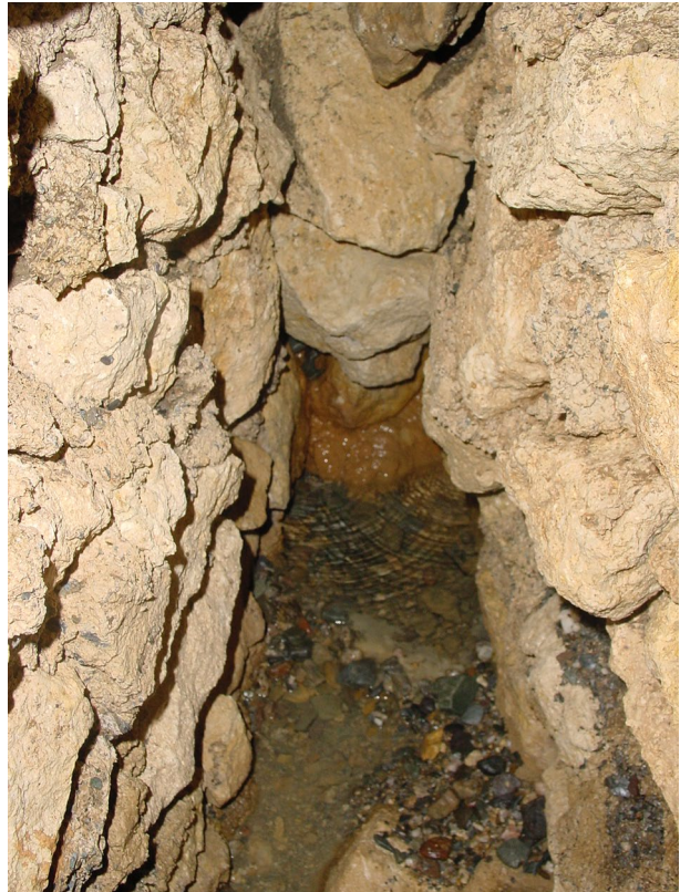
Fig. 7 Hole in the wall ( mechinal, piquera o tronera ) of the preceding filter gallery to the groundwater dam of the Contracaño (Puerto Lumbreras, Murcia)
