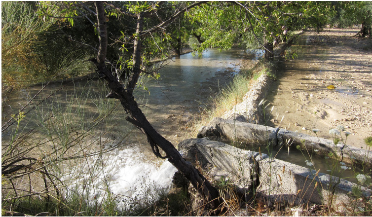
Fig. 4 A typical irrigation canal in the Vega of Vélez Blanco, which conveys water from an upper to a lower olive field. The former earthen canals were renewed with concrete modules in the 1960s
