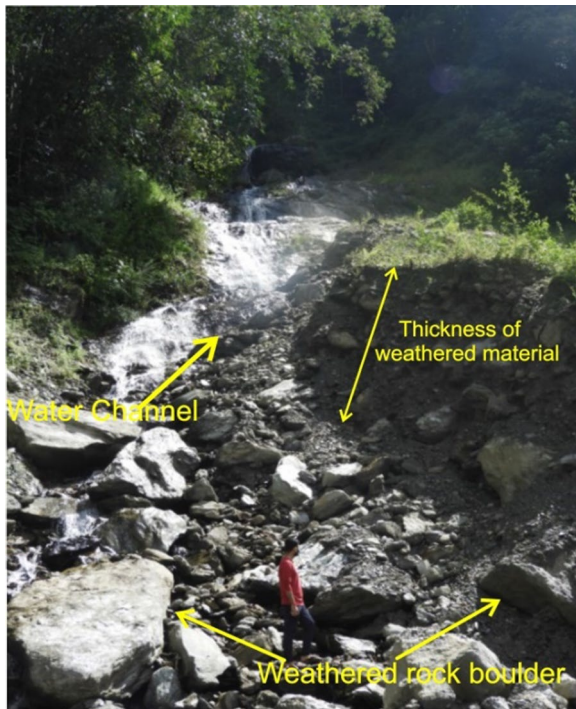
Fig. 7 Presence of surface water or flowing channels of water contributes to the occurrence of slope failure
