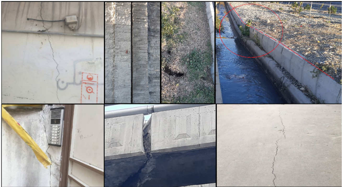
Fig. 8 The effects of land subsidence on various urban elements in the study area
