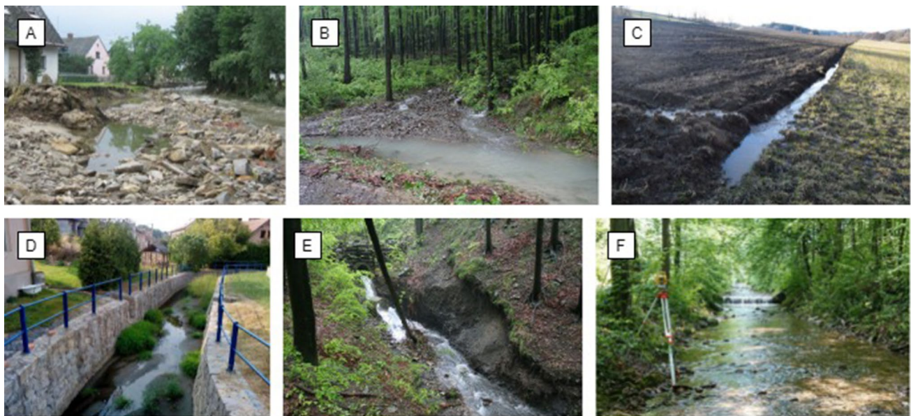
Fig. 1 Examples of critical issues associated with sediment transport management in mountain streams in Czechia. Conditions of sediment excess (photos A–D) and sediment scarcity (photos E–F). A Severe sediment accumulation during floods in inhabited areas, B jamming of culverts and flooding of roads during flood events, C supply of fine sediments from agricultural land to coarse-bedded streams and rivers, loss of physical habitats (e.g. fish-spawning gravels), D sediment
