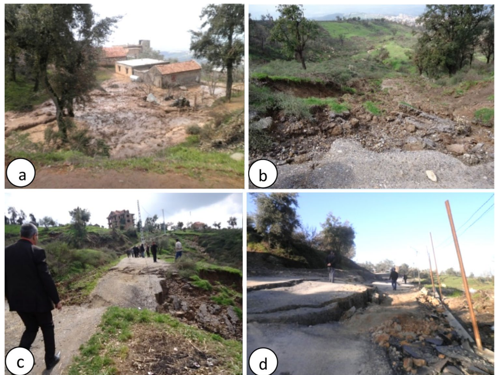
Fig. 1 Examples of different types of landslides induced by the March 12, 2012 rainfall event in the city of Azazga: a debris flow and damage to constructions in Agouni Guizem, southeast of the city, b debris flow along the Boulina river, south of the city, c damages of municipality road in the Agouni Guizem, d damage along national road RN 12 in Ighil Bouzel and Zen, north of the city
