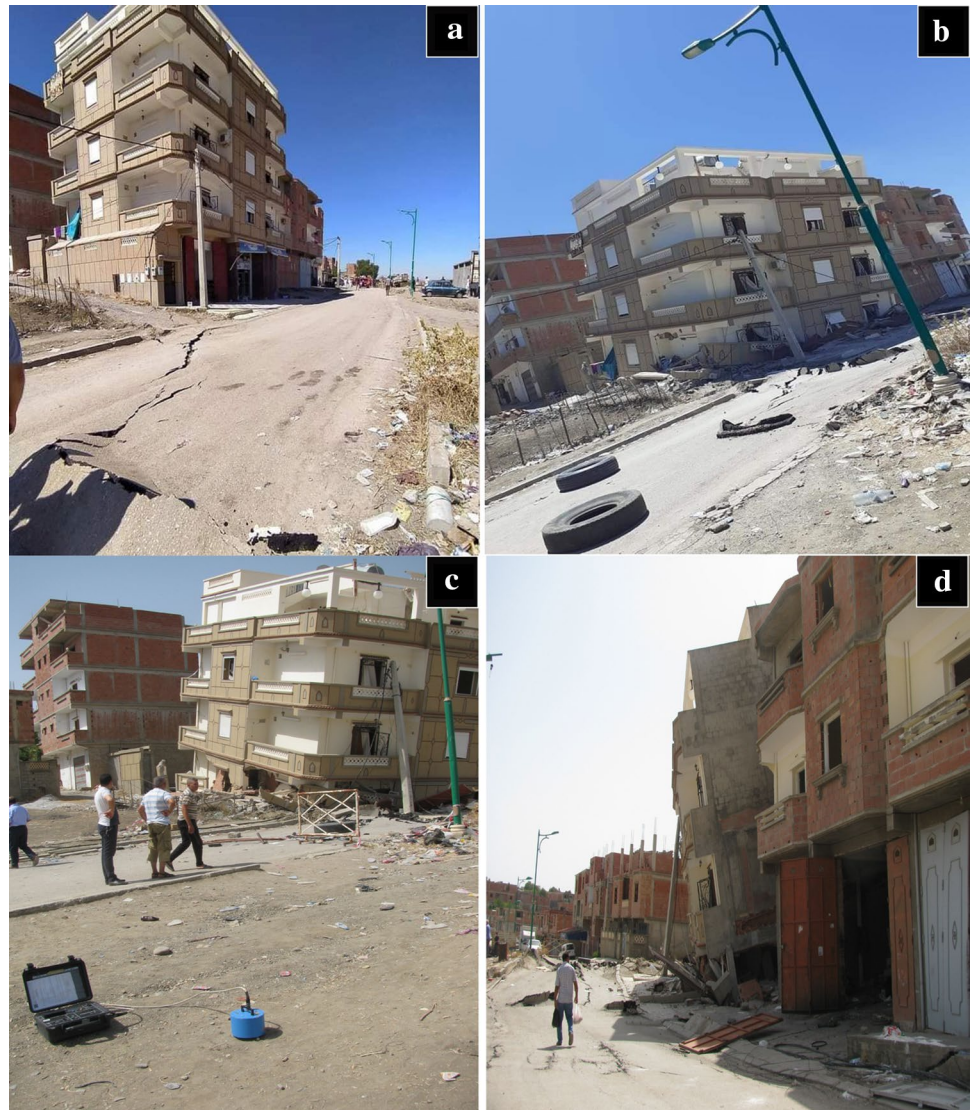
Fig. 7 Example illustrating landslide evolution showing the tilting and sinking of a building
