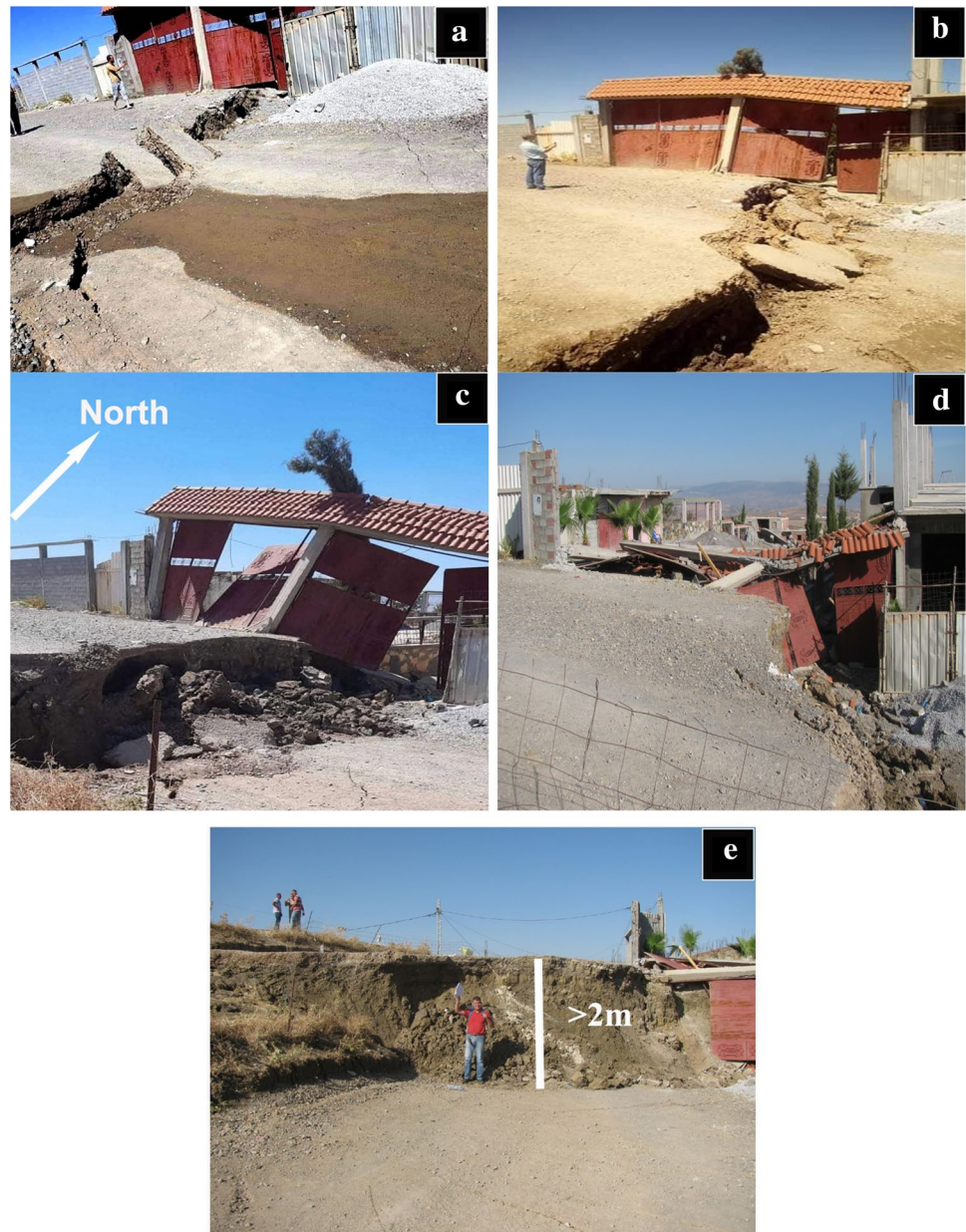
Fig. 6 Evolution of a lateral scarp from a centimetric a to a metric e vertical displacement affecting an entrance gate that tipped and then was buried in the ground
