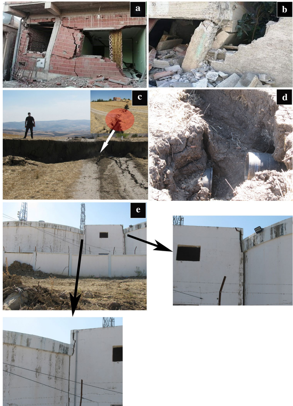
Fig. 3 Photos a, b show the damage caused by the landslide to the structural elements of the houses, c Subsidence and horizontal displacement of a road, d Rupture of a sewer pipe, e cracks in the water tower and increase of the opening at the rupture joint
