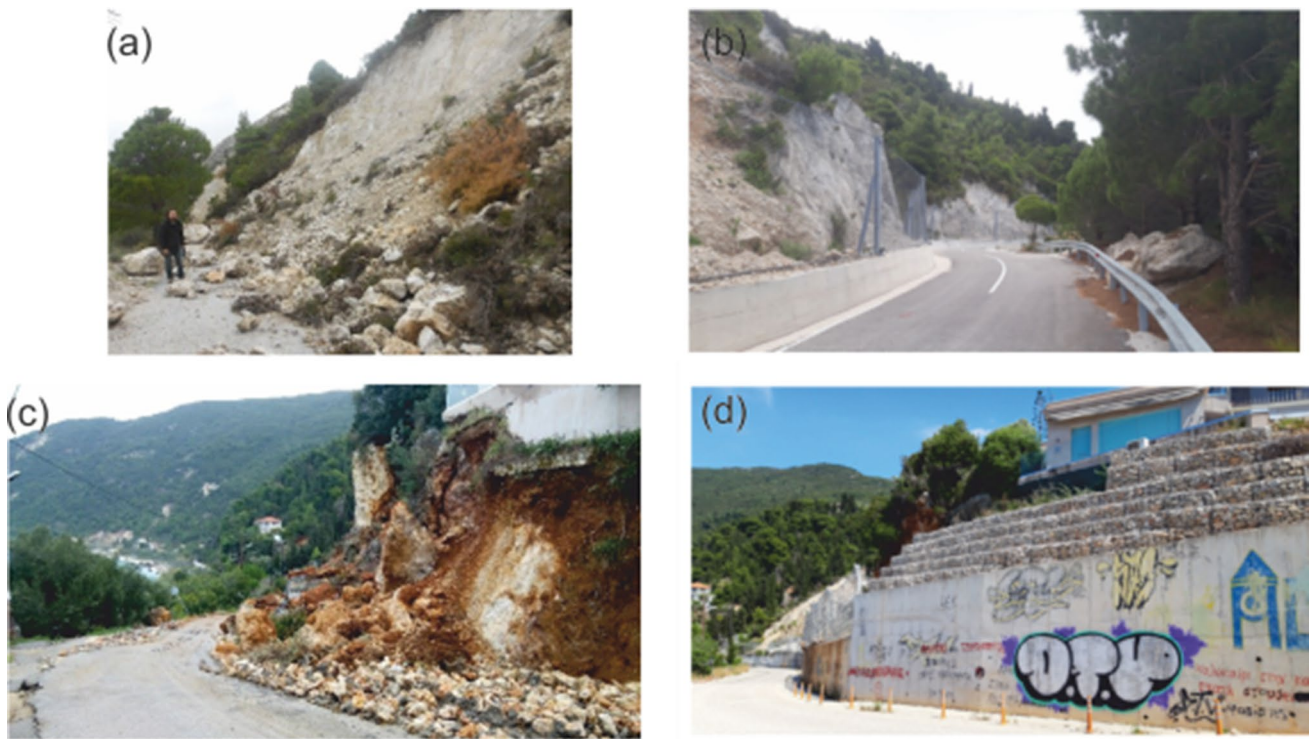
Fig. 2 Comparative pictures showing: a Rock slide at the area of Gialos (photo taken on November 21th, 2015), b rockfall protection mesh at the same area (photo taken on May 26th, 2020), c rockfalls in the
