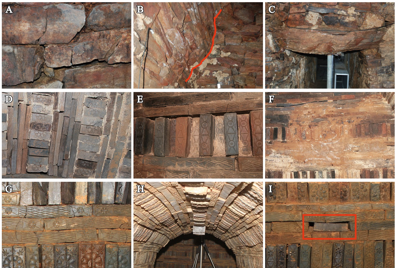
Fig. 3 Present status of the Royal Tombs at Songsanri ( a–c tomb no. 5, d–f tomb no. 6, g–i Royal Tomb of King Muryeong): a structural cracks and fractures in the rock. b Swelling phenomenon on the west wall. c Subsidence of the large horizontal member due to loading. d Cracking, separation, and distortion concentrated on the ceiling. e
