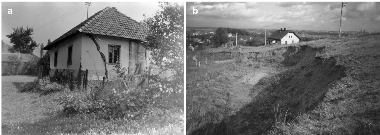
Fig. 18 Sladaja village: a Damaged object above the old exploitation works of the “Strmosten” pit; b Surface subsidence above the actual exploitation works in the “Strmosten” pit
