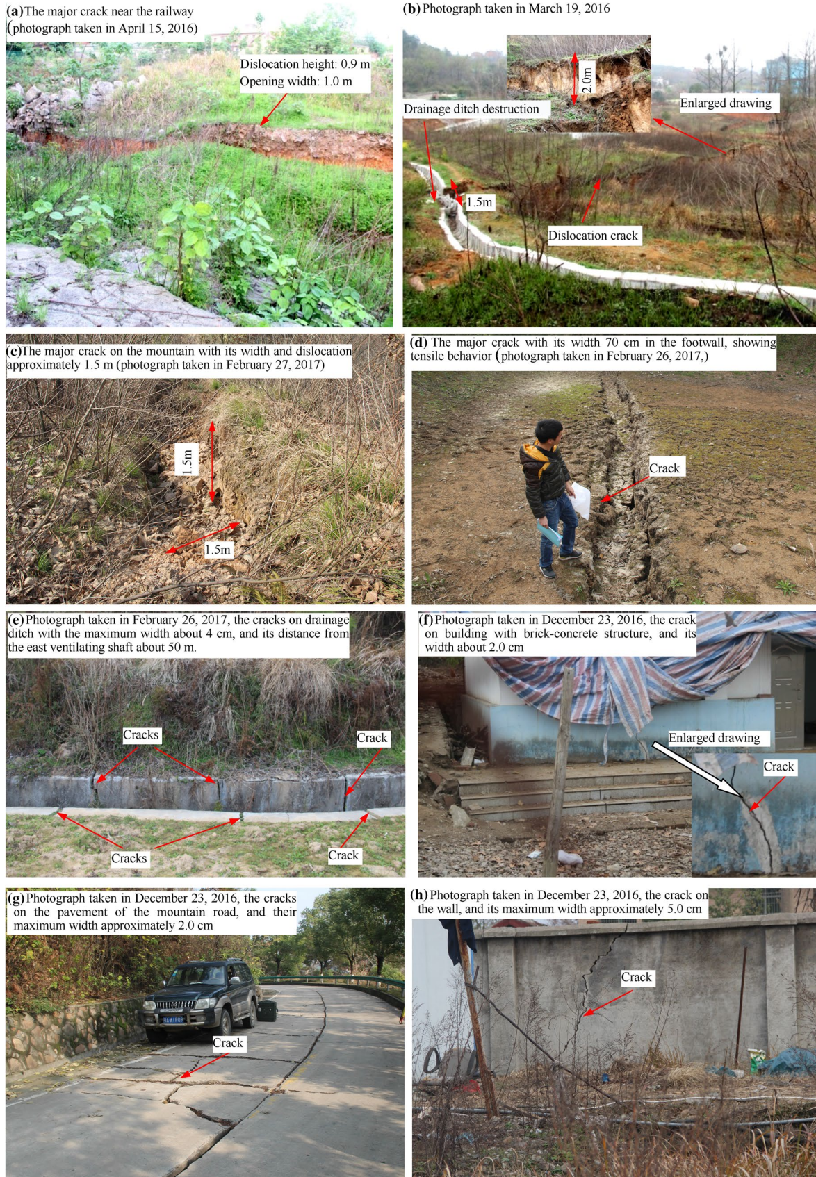
Fig. 8 The cracks on the ground surface, the buildings and facilities (the location of these cracks is seen in Fig. 6)
