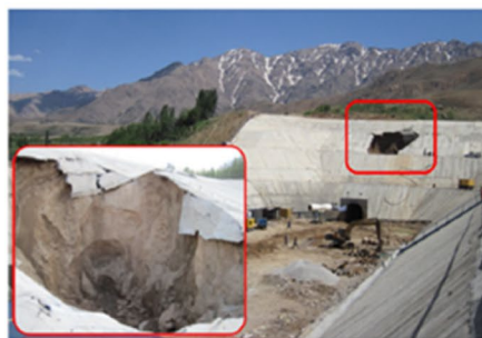
The first collapse
