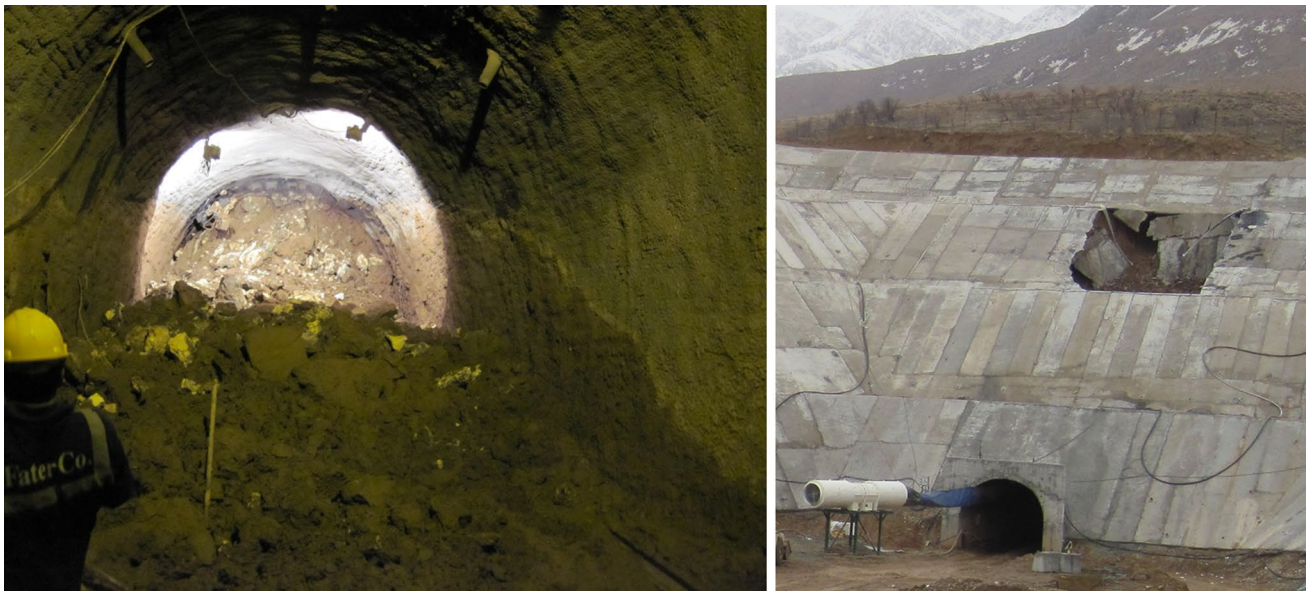
Fig. 5 The first tunnel collapse occurred in the northern portal of Sabzkouh tunnel (Eftekhari et al. 2014)
