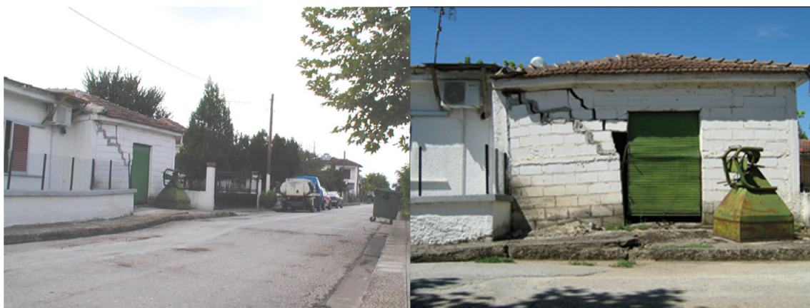
Fig. 2 Damages due to land subsidence in West Thessaly basin. The cracks in the stonework on the left photo by Apostolidis and Georgiou (2007) evolve, despite the repairs even 8 years after, as seen in the right photo taken by the authors (2015)
