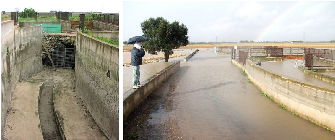
Fig. 3 The entrance of Vora Colucce; left: in dry condition at the end of a channel cleaning work (July 24, 2006); right: a flood event (December 4, 2008) resulting from an intense precipitation occurred the day before (see Table 1)
