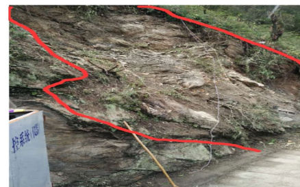
(a) The slight landslide that occurred on September 24
