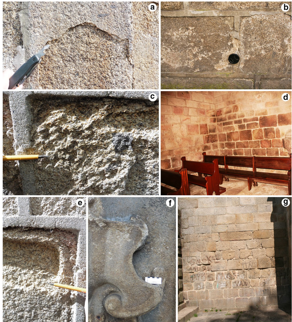
Fig. 1 Example of weathering forms on granitoids: scaling (a), black crusts (b), pitting (c), oxidation (d), alveolization (e), missing part (f) and graffiti (g)
