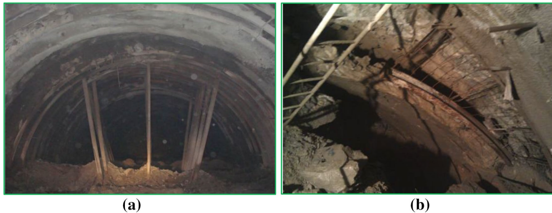
Fig. 6 Failure of the tunnel in squeezing rock a large deformation b damage of the primary lining
