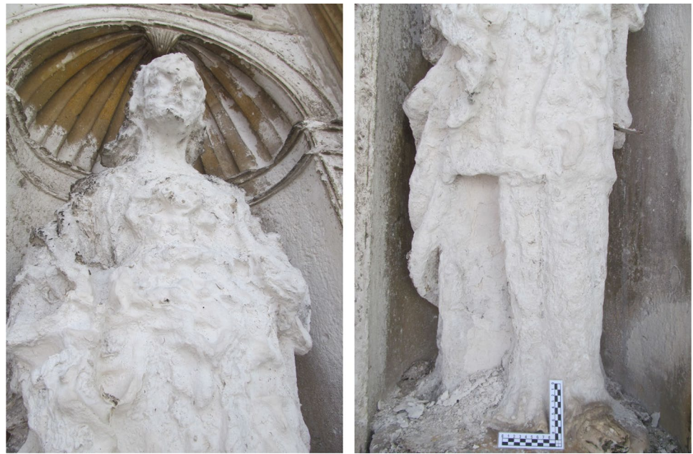
Fig. 4 Details of pathologies of Medicine statue (4E) on the East portal showing powdering and scaling
