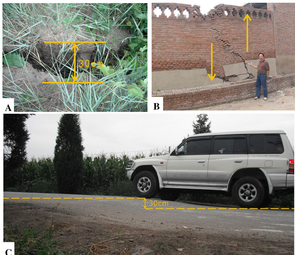
Fig. 14 a Ground surface cracking due to fissure f_3 ; b damage to a building in Xiguan village due to fissure f_3 ; c vertical differential settling of the road due to fissure f_3 . The location of each picture is indicated in Fig. 6
