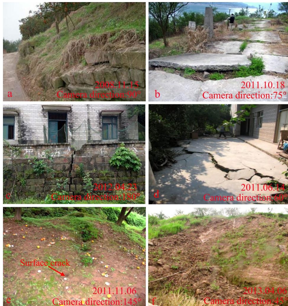
Fig. 5 Deformation and damage characteristic photographs from the study area
