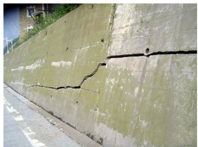
Fig. 4 Earthquake damage cases
