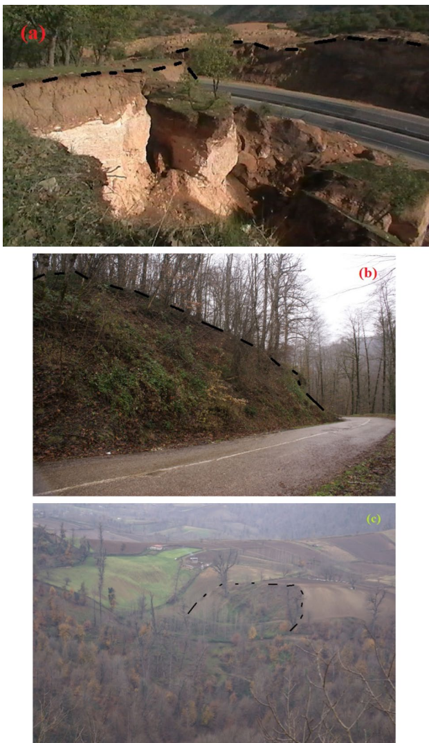
Fig. 3 Field photographs of some identified landslides in the study area
