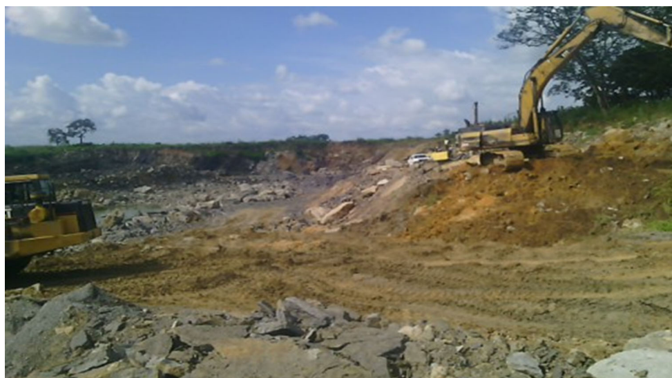
Fig. 8 Excavated land area and vegetation loss in Amaeze Community
