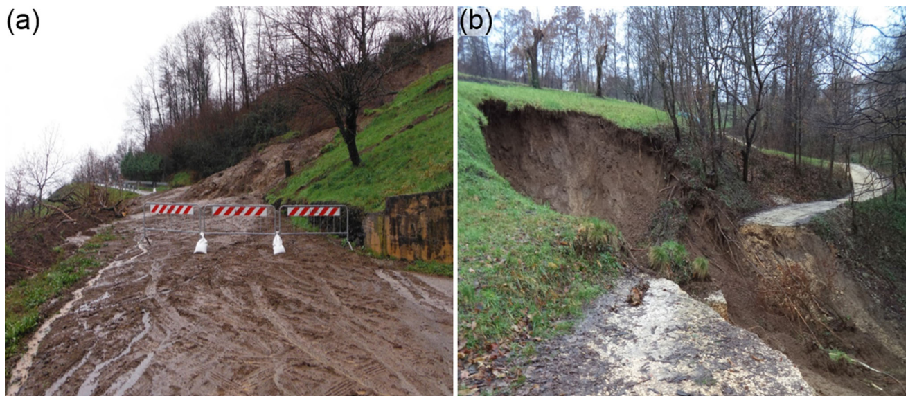
Fig. 3 Typical landslides occurring in the study area: a earth flow, b rotational slide/flow. In evidence the damage to the road network
