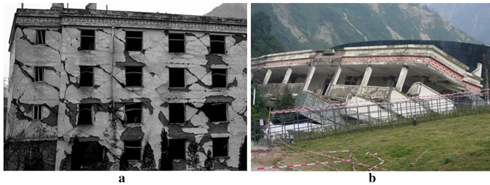
Fig. 21 The seismic damages of the superstructure. a Framework structure. b Frame masonry structure
