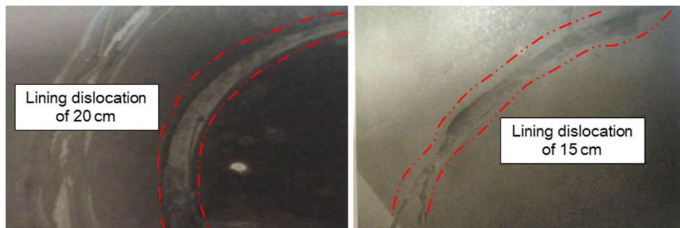
Fig. 14 The lining structure dislocation (Mao et al. 2011)
