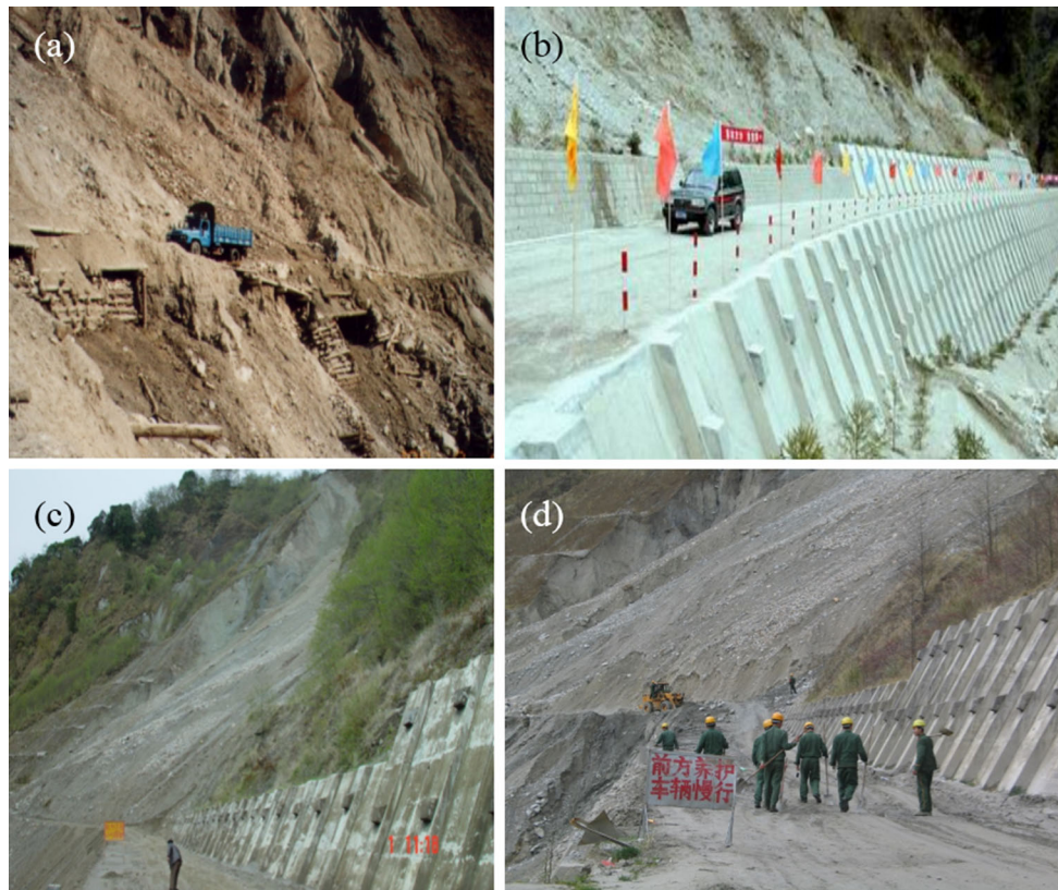
Fig. 11 Evolution of the 102 Landslide to form gully divisions between 2001 and 2006: a wood retaining wall for basement reinforcement (February 2001); b reinforcement of the highway surface to ensure traffic safety at a cost of 53 million yuan (December
