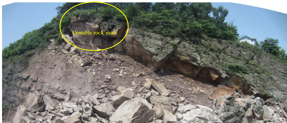
Fig. 3 Photograph of rock slope after second failure (on April 29, 2014)
