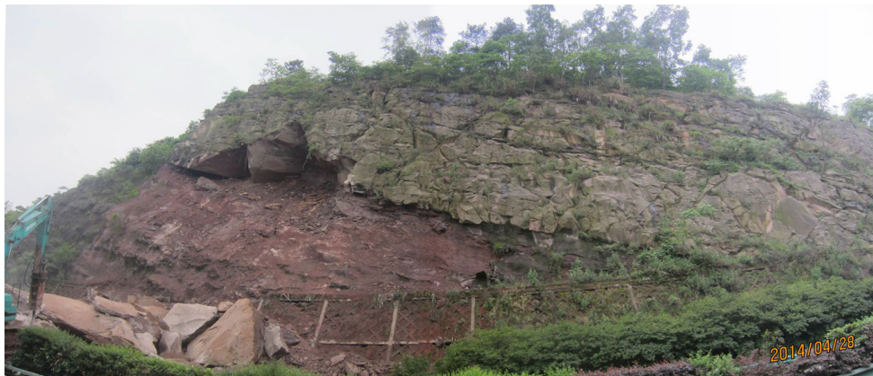
Fig. 2 Photograph of rock slope after first failure (on April 28, 2014)
