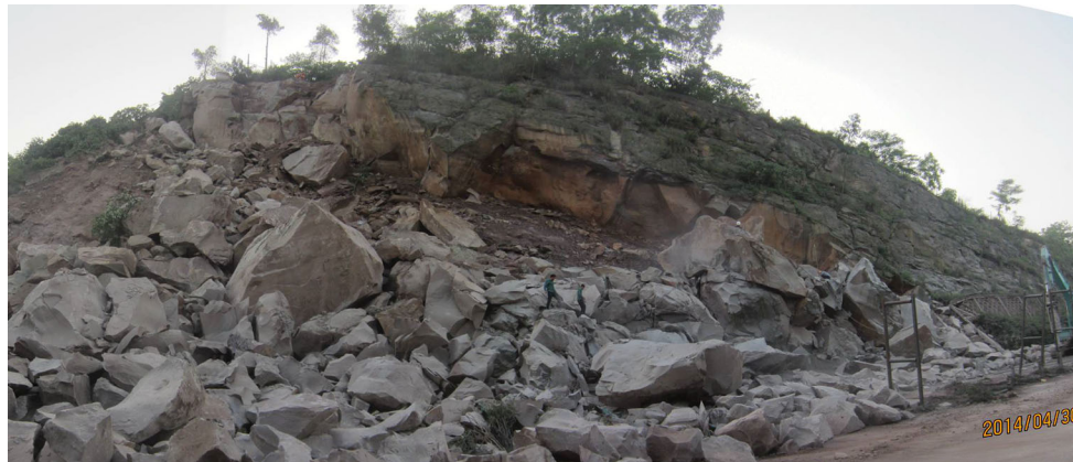
Fig. 4 Photograph of rock slope after excavation of unstable rock mass (on April 30, 2014)
