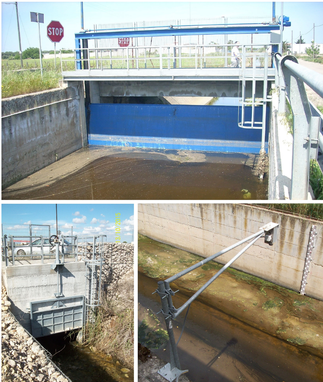
Fig. 8 Above the sluice gate SA along LB1 is closed to drain Asso Torrent toward the sea through LB2. Below on the left the gate SB is regulated for a low flow in LB1. Below on the right the hydrometer H monitoring helps the decision making
