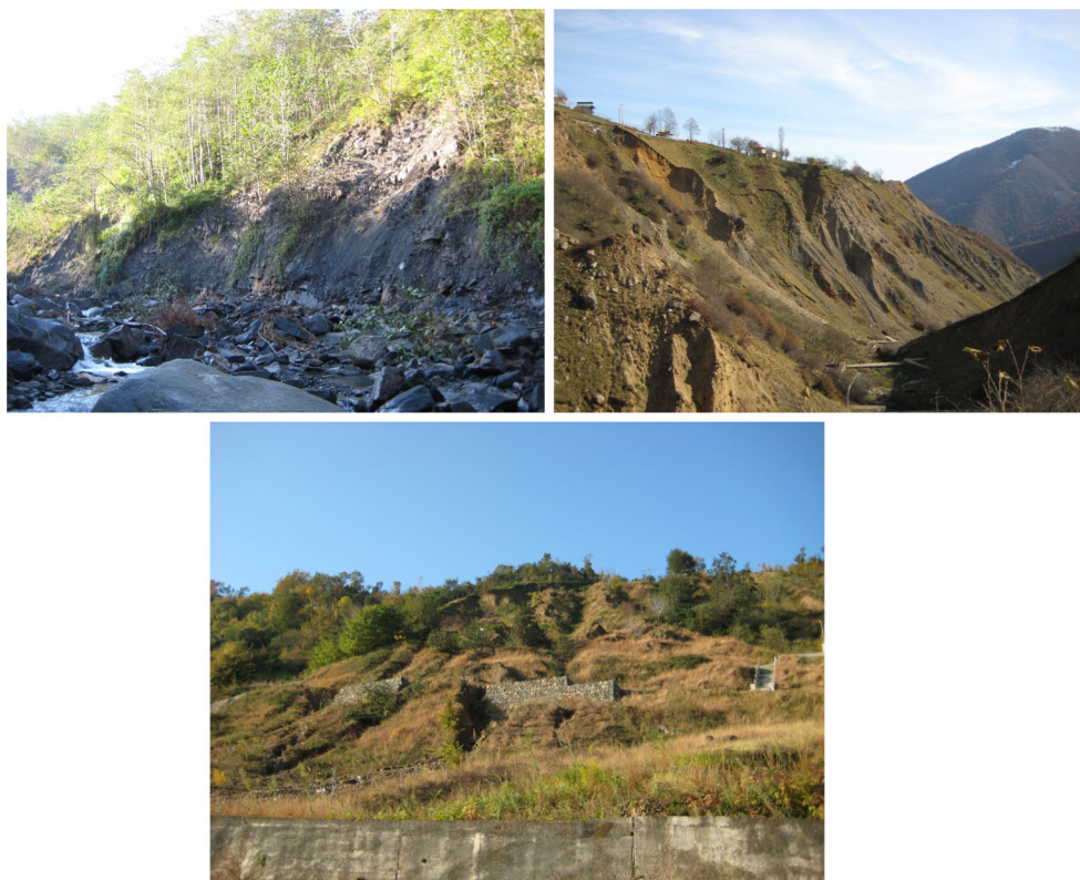
Fig. 3 Field photographs of some identified landslides in the Safarood Watershed
