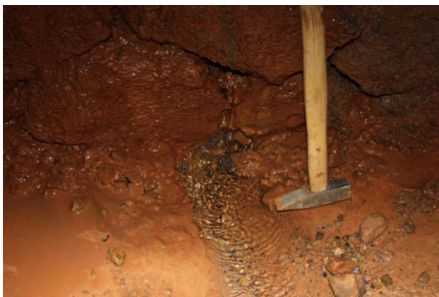
Fig. 6 Runoff of groundwater near the slip zone
