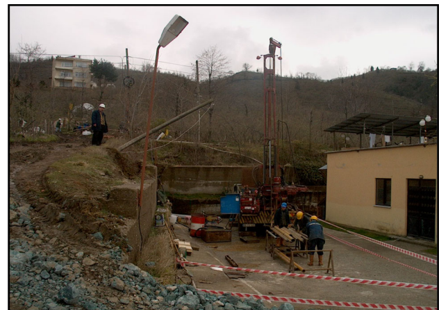
Fig. 9 A view showing Tünel restaurant (to the right) and the tilted retaining walls after the occurrence of the landslide (to the left)
