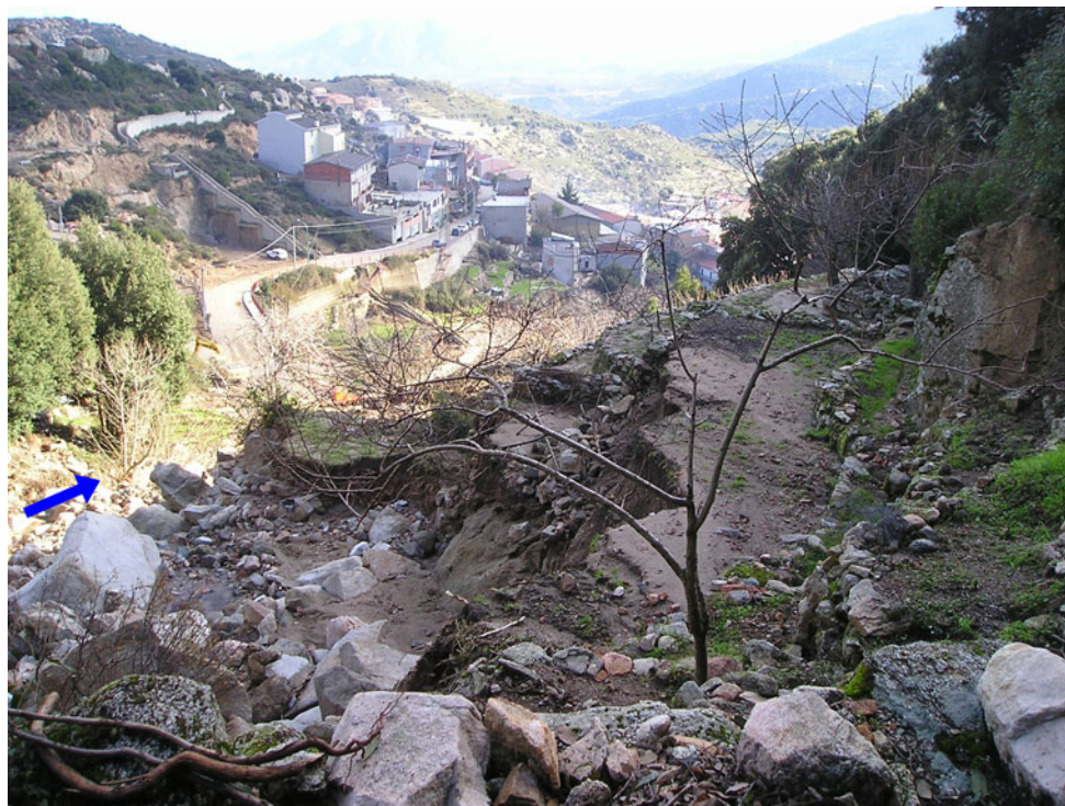
Fig. 4 In the lower catchment sectors in vicinity of the housings, widely diffused, privately owned kitchen gardens, sustained by typical man-made stony walls, were partly invading the flood cross-section of the torrent. Several shallow slides just originated in such
