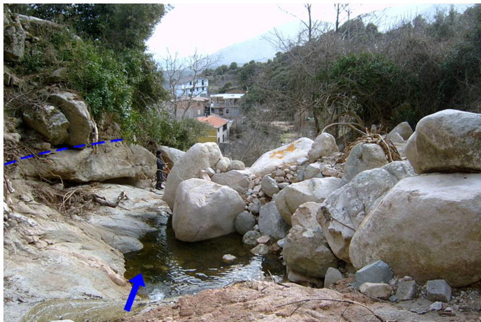
Fig. 3 At the catchment head of the Bau Argili torrent, the dimension of the blocks set in motion by the 2004 flood also exceeded 2 m. Stream-bank erosion ( left on the picture) has removed the uncohesive
