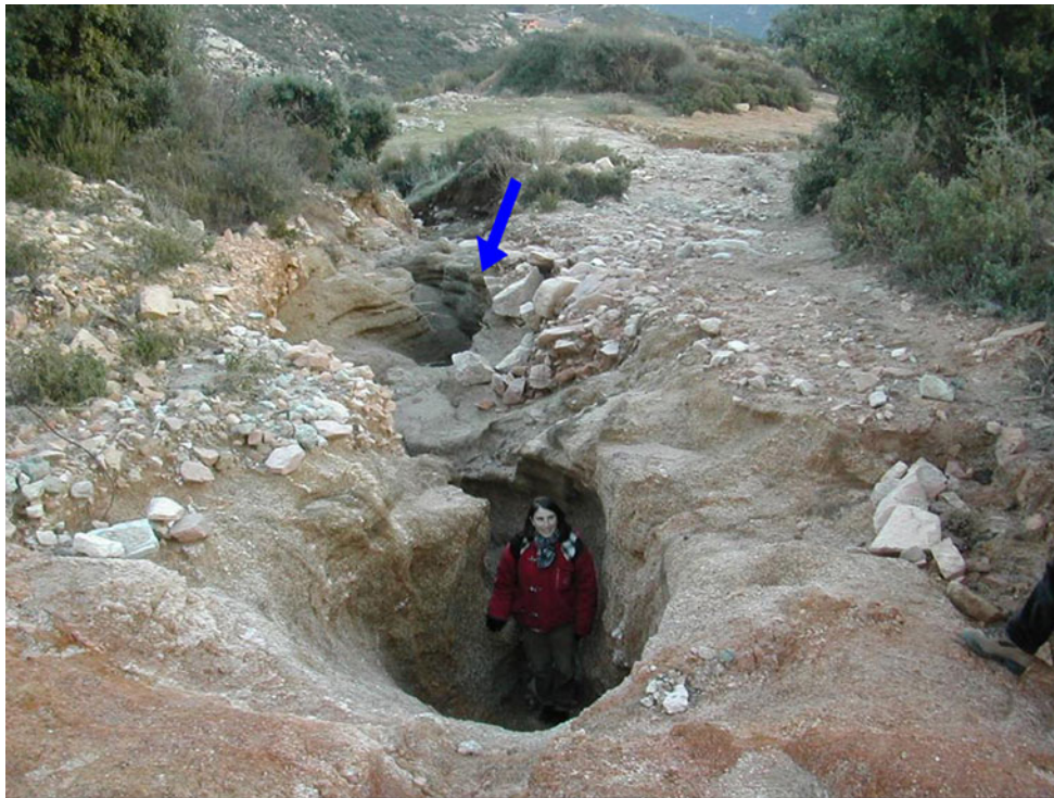
Fig. 5 Gully erosion in a forestry track above the Villagrande village ( Serra e' Scova catchment), produced by intense runoff. In the uppermost part of the village, erosion phenomena are particularly apparent along streams and forestry tracks. As a matter of fact, most
