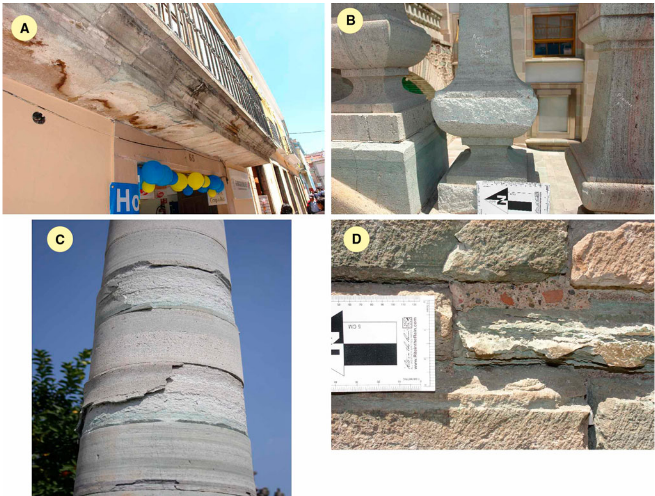
Fig. 2 Appearance of the different damage and deterioration types observed in the Loseros Tuff. a Flaking in the lower parts of a balcony. b Crumbling in the bars of the staircase of the university.
