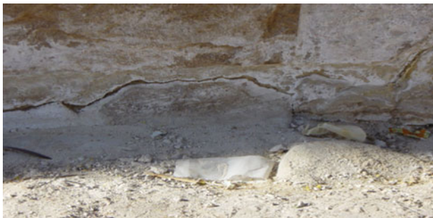
Fig. 2 Effects of shallow saline groundwater on the Habu temple (note the severe cracks and salt accumulations)
