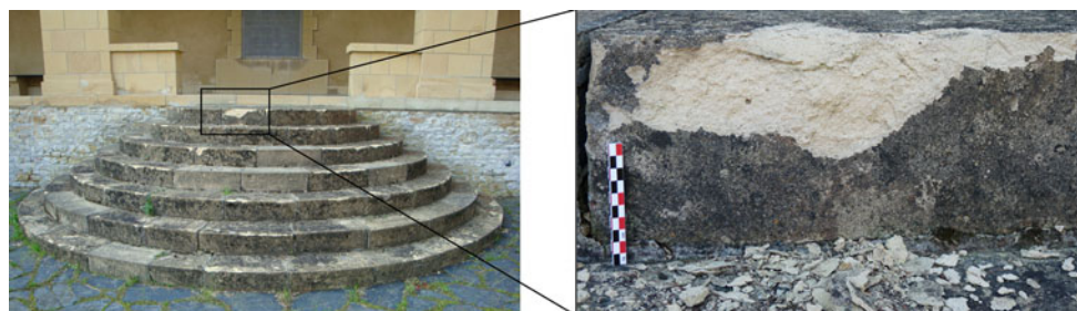
Fig. 4 Typical patterns of frost damage on reconstituted stone viewed on the stairs of the cemetery: cracking and chipping of blocks
