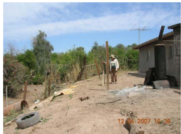
Fig. 6 Photograph of site F1 (Fig. 2) showing the Saltillo fault where the crackmeter is installed as seen from the S. This place was flat in the beginning of the 1970s
