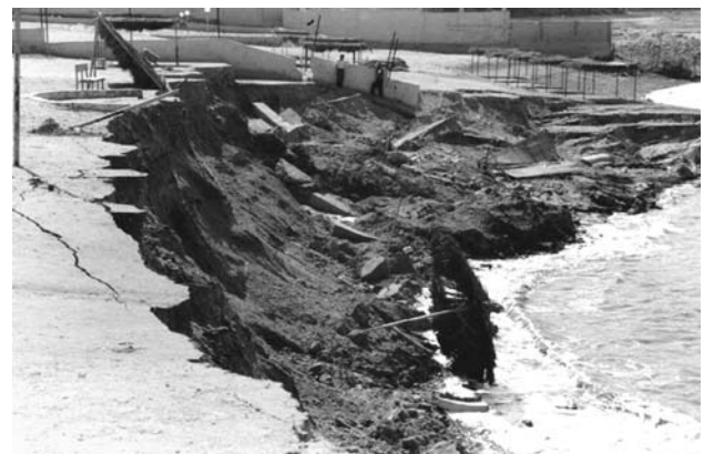
Fig. 5 September 6th, 1999, part of a touristic beach at the northern DS was destroyed by a sudden ground collapse. In 2004, a decametric sinkhole occurred close to the wall where people were looking at the scarp ( upper middle ). From 2006, the whole area was included into the perimeter of the private beach of a new five-star resort (Holiday Inn). The scarp was covered by a stone wall. In May 2007, the wall collapsed partially. In May 2008, three salty springs were found along the seepage surface (the beach). They attest that water is flowing below the hotel and its surroundings, continuing to dissolve salt remains
