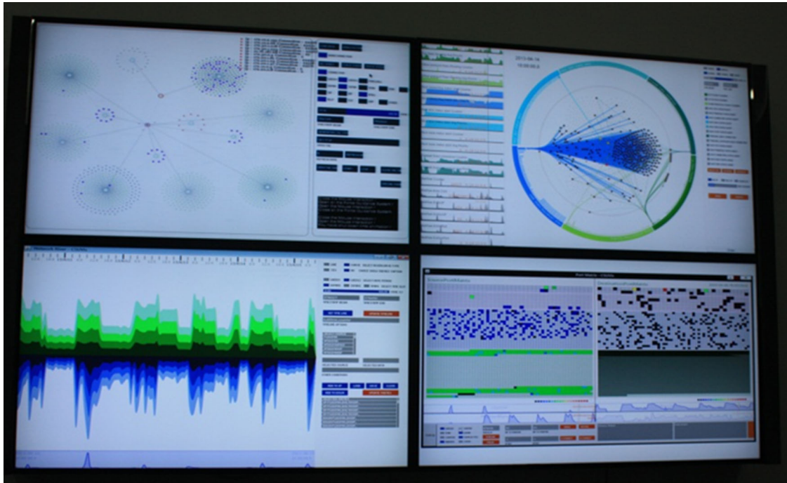
Fig. 13 Using system with four tied displays in the control room
