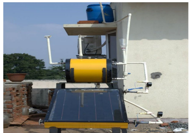
Fig. 1 Experimental set-up of solar water heater
