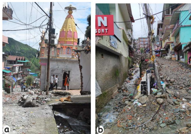
Fig.5 (a) A temple constructed right on top of the Bhagsu nala and (b) view of the constricted drainage towards the lower reach of the Bhagsu nala.
