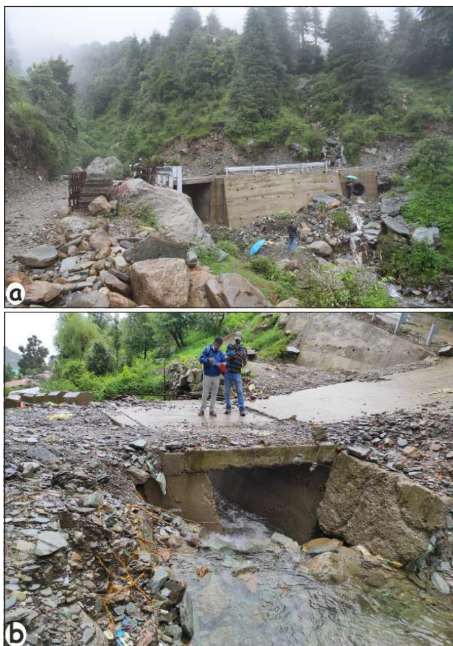
Fig. 4. (a) View of the Bhagsu nala looking upstream (b) View of the culvert reducing the carrying capacity of the Bhagsu nala
