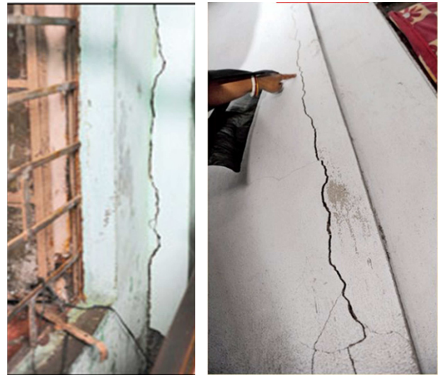
Fig.19. Observed cracks in Ultadanga police quarter (BH 130) during 2011 Sikkim earthquake ( www.ndtv.com )
