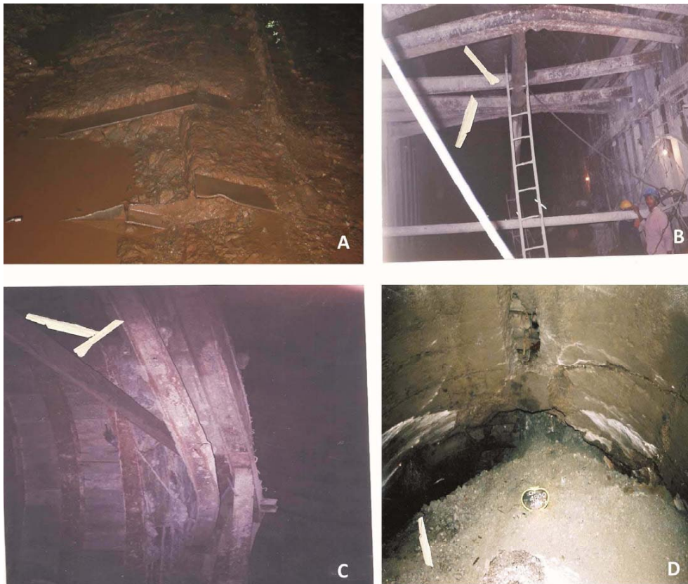
Fig.1. The effect of lateral displacement and deformation of ground on tunnel’s support system; (A) Invert heaving, (B) Buckling of cross-strut, (C) Buckling of ribs, (D) Partial collapse of crown
