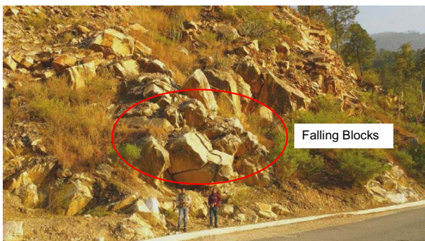
Fig.3. Rockfall along the road cut section
