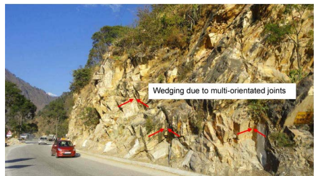
Fig.7. Road cut section shows wedge failure
