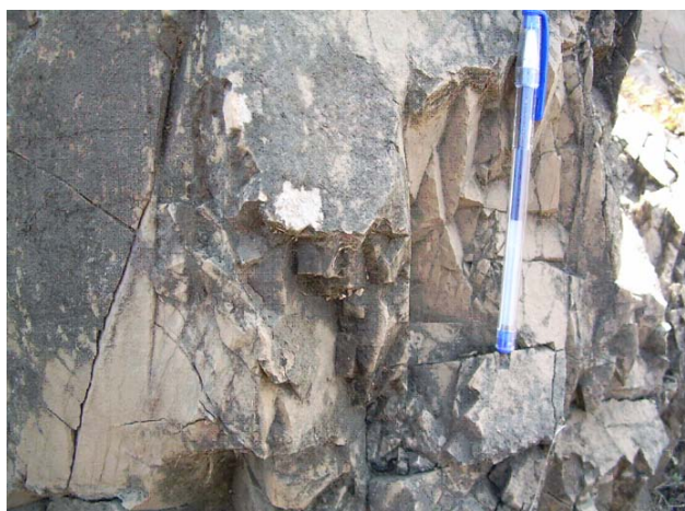
Fig.11. Shear zone rock i.e. hard phyllite/mylonite is showing very high degree of fracturing.
