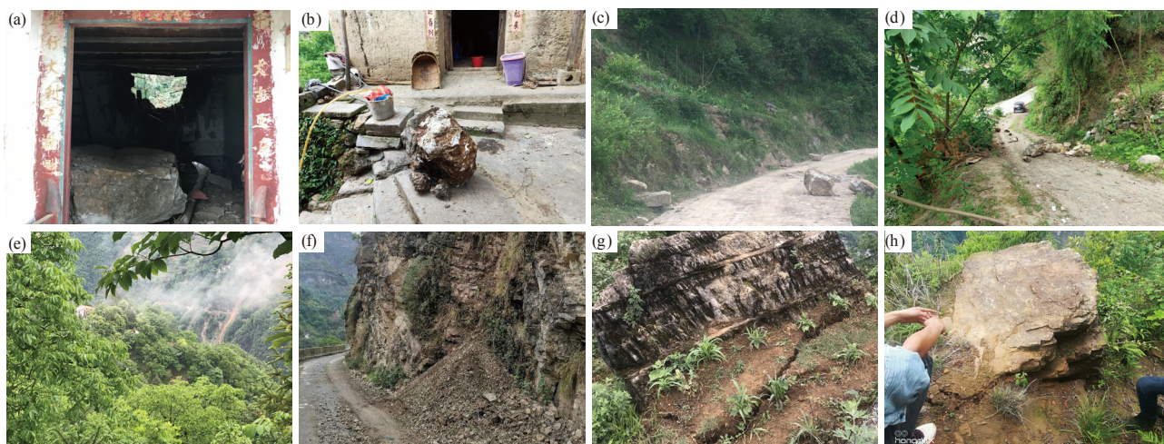
Figure 2. Pictures showing landslide hazards during 2020 Qiaojia earthquake. (a) and (b) damaged houses by rockfalls; (c) and (d) blocked roads by rockfalls; (e) and (f) debris slides; (g) and (h) imminent falling rocks with ruptures.
