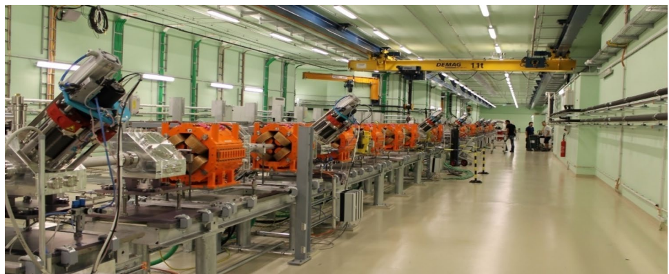
Fig. 7 The high energy transfer line HEFT delivers the beam to four irradiation rooms. Quadrupole magnets are noticeable (orange color) and the scintillating fiber hodoscopes (SFX) beam monitors are also visible (red and blue)
