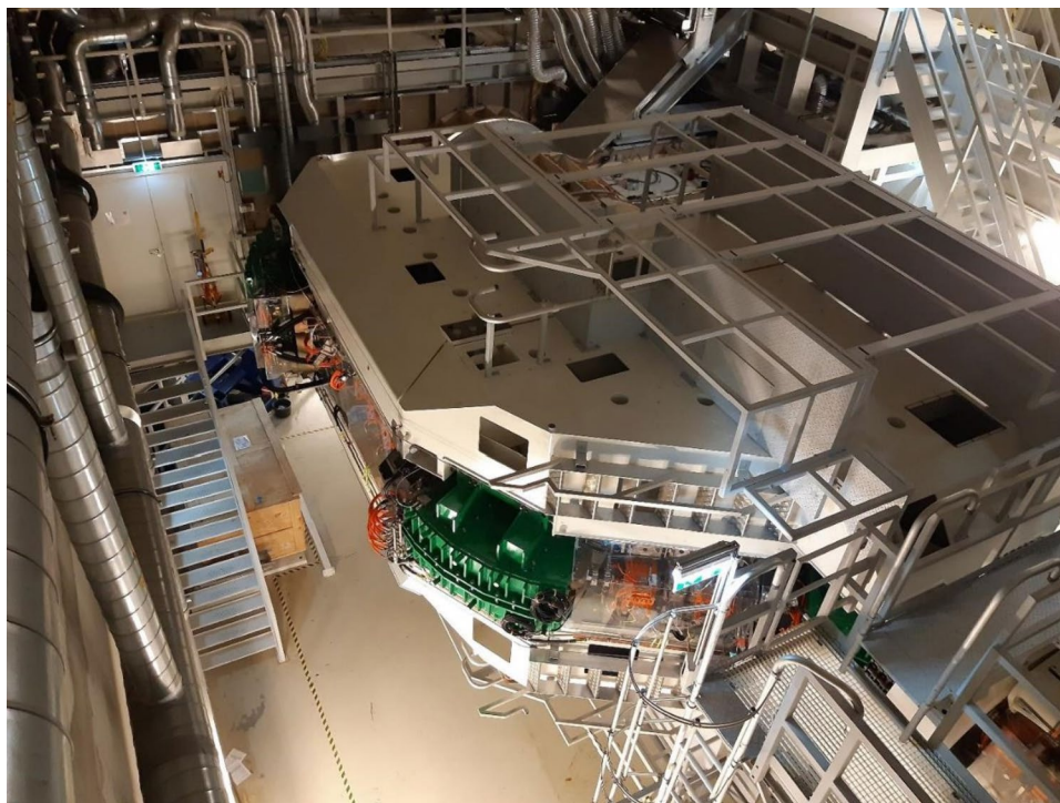
Fig. 9 Bird view of the MedAustron proton gantry laying in the horizontal position (gantry rotation angle 90^\circ ). The beam entrance into the gantry beam line is on the lower-right corner while the patient irradiation room is located behind the wall on the upper side of the picture
