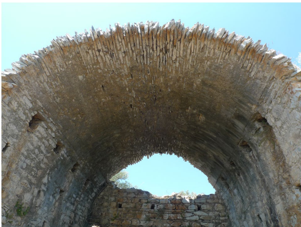
Fig. 13 Roman stone barrel vault at Iasos (Turkey) made with thin stones placed radially
