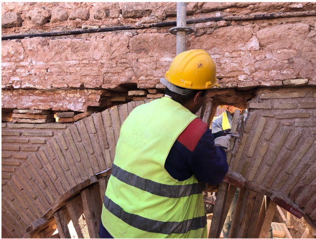
Fig. 4 Construction of a brick arch with rectangular bricks (Chellah, Morocco). The wedged shape of mortar helps in giving a radial disposition to the bricks
