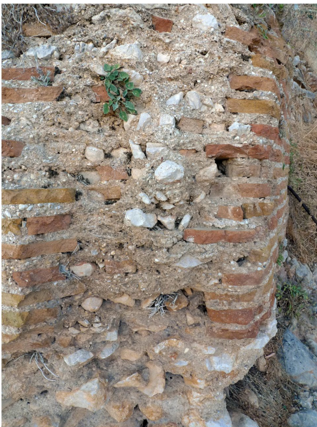
Fig. 11 Brick-faced rubble masonry wall of the Roman aqueduct at Argos (Greece). The mortar joint is 2 cm, while the bricks are 4 cm thick. The many hollow spaces in the nucleus show little attention to reaching high compactness in the masonry
