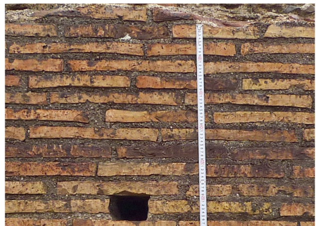
Fig. 3 Brick-faced Roman concrete (Argos Aqueduct, Greece). Differences in thickness and form of the brick are compensated for by the mortar joint
