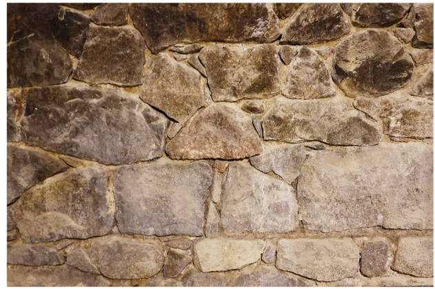
Fig. 2 Masonry with large granite blocks (larger blocks are 50×80×33 cm) and small stone flints placed at the joints (Kizer House, South Bend, IN). Mortar joints are minimal and stresses are transmitted principally through contact points
