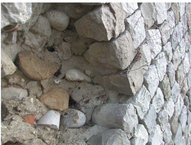
Fig. 7 Failure of an opus reticulatum facing because of the poor bond with the core of the wall. The soundness of the masonry is diminished by the use of river stones and the many hollow spaces in the masonry (Herdonia, Foggia, Italy)
