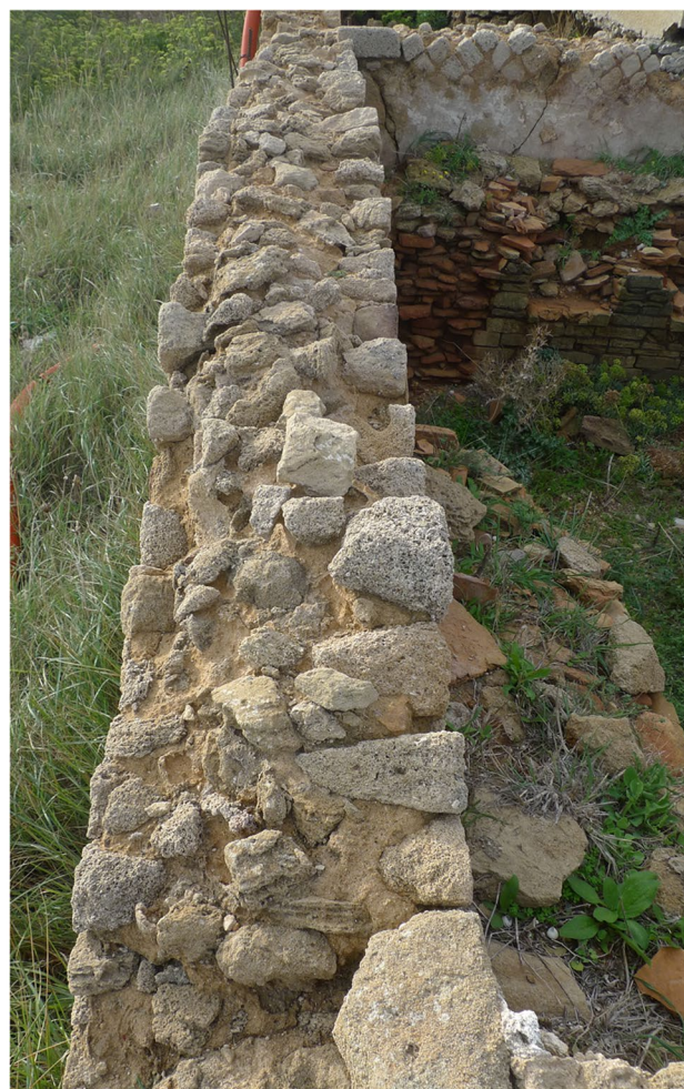
Fig. 6 Opus reticulatum wall in Capocolonna (Crotone, Italy). The two facings are made with stones cut in pyramidal shape so as to reinforce the bond with the core. Mechanical properties of the wall may decrease if the masonry is roughly assembled
